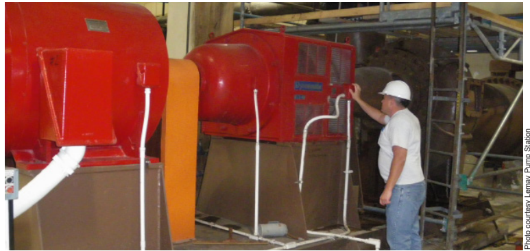
Photo courtesy Lemay Pump Station
